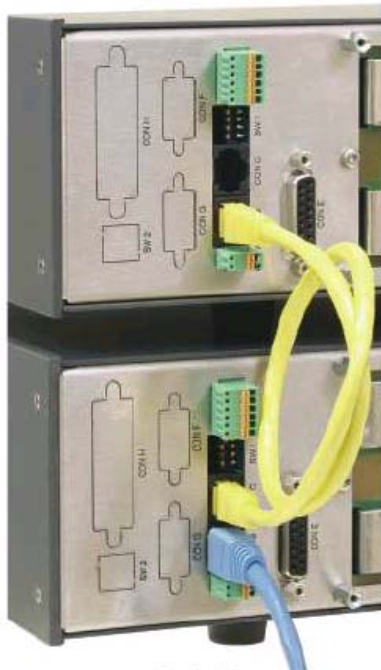
Fig 3 - 22 Use standard UTP cables (RJ45) for Master / Slave operation
